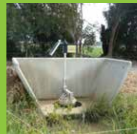
Automated outlet riser from a pipe source.
